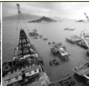
Aviation fuel facility jetty at Chek Lap Kok airport, Hong Kong
